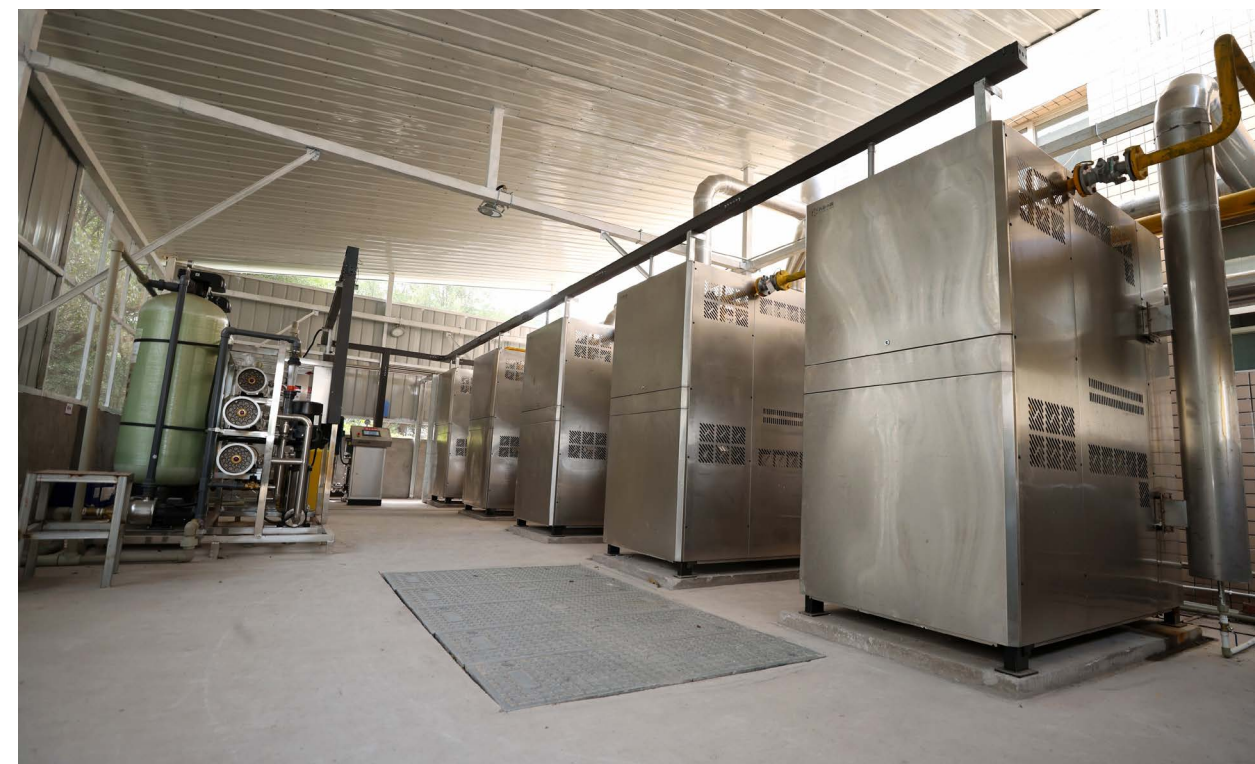
▲ Steam module generators in ZCC
