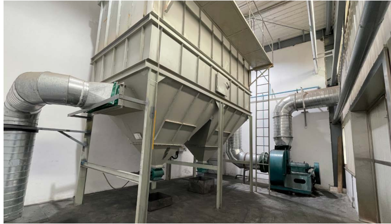
▲ Wastewater treatment facility in ZCC CT
